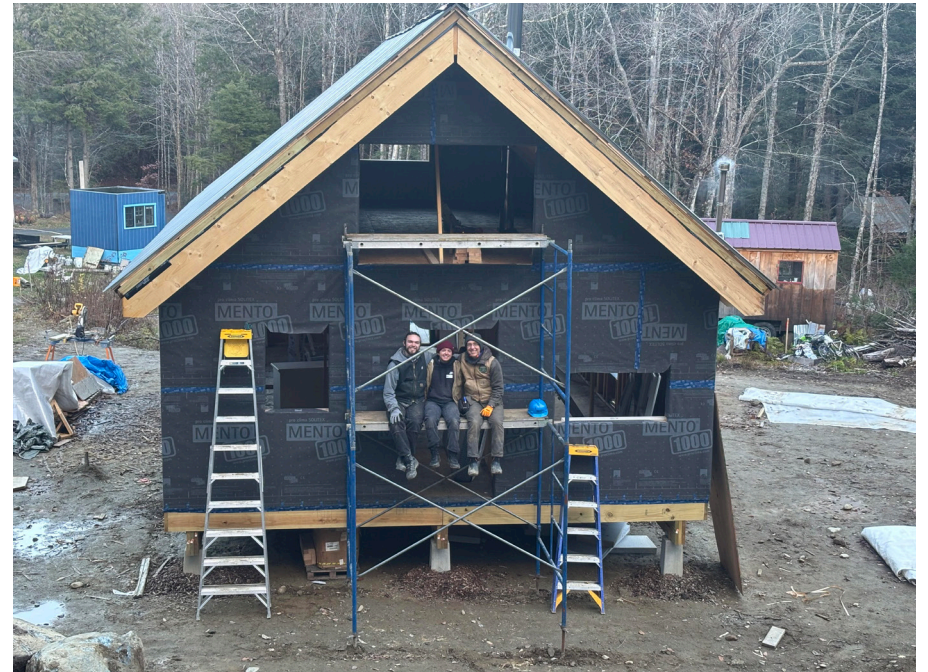
The Dandelion Housing Project team working on a cabin. Photo credit: Murphy Robinson
